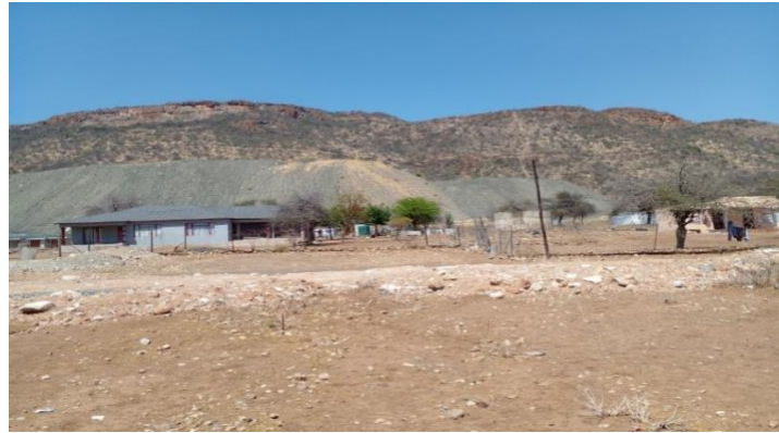
Blast vibrations causes damages in homes near Bauba Platinum Mine
