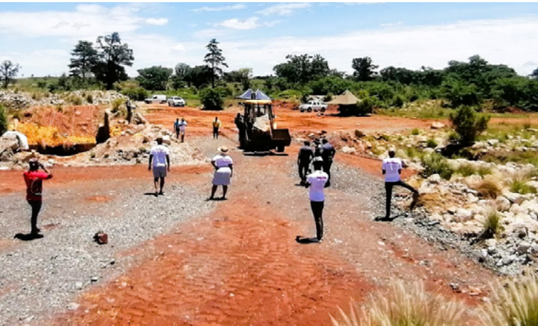
Stilfontein Solidarity Committee hired a Grader to repair the pulley system damaged by Police and Buffelsfontein mine.
